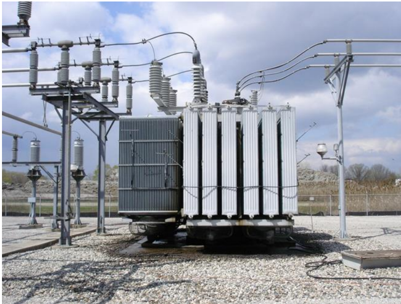
Exhibit 8.1.1 Typical Substation Power Transformer
