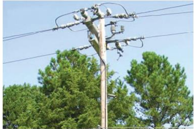
Bridges Auto Topper switches
