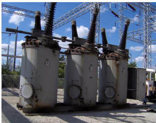
Traditional 120 kV Oil Breakers
