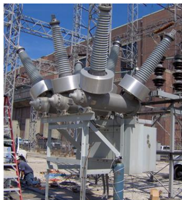
Modern 120 kV Gas Breakers
