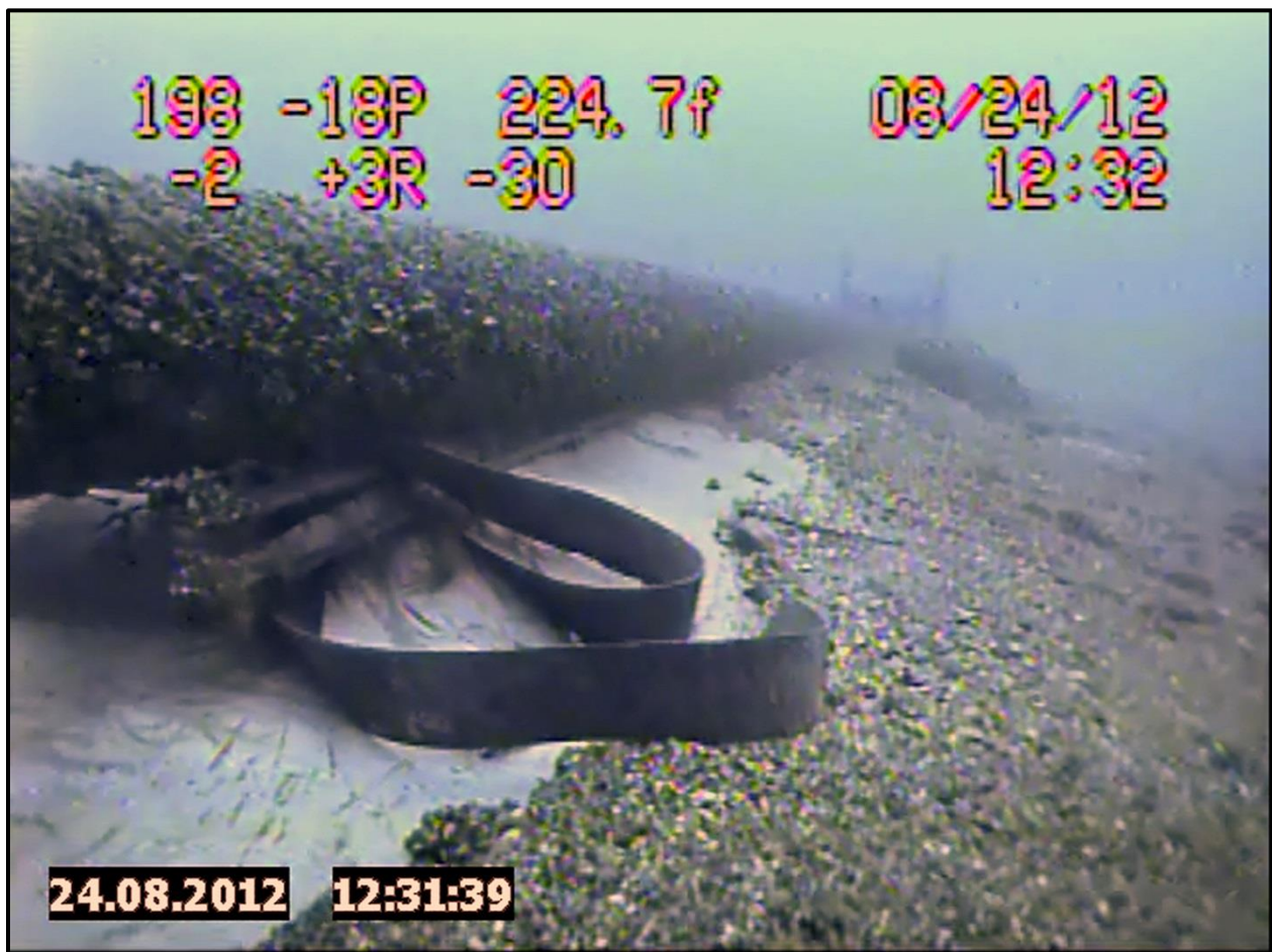
Figure 5 Broken Lifting Strap around West Leg from 2012 Enbridge Inspection Video
