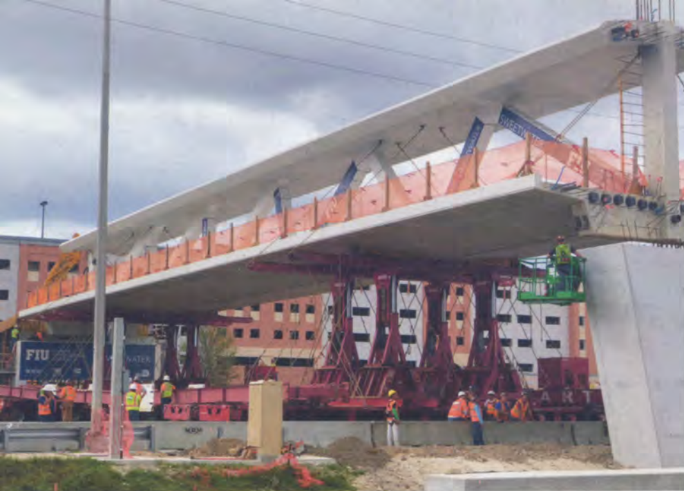
The Miami bridge was designed to look like a cabled-stayed bridge but departed from the usual construction schedule of such structures by having its deck (the pedestrian walkway) hoisted and moved into place before the cables and towers were erected.
