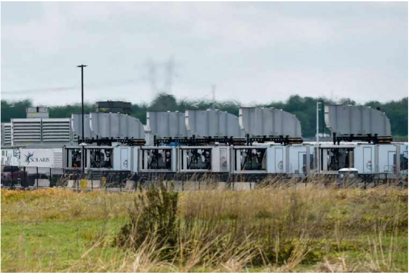
Gas turbines are visible at the xAI data center on April 25 in Memphis, Tenn. Credit: Brandon Dill/The Washington Post via Getty Images
