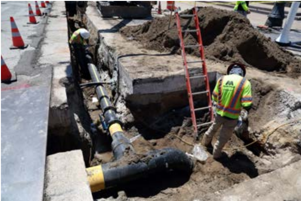
Juan De Luna, left, and Lino Banuelos, from Miller Pipeline, put the finishing touches on a section of a Peoples Gas pipeline replacement project at Wrightwood and
