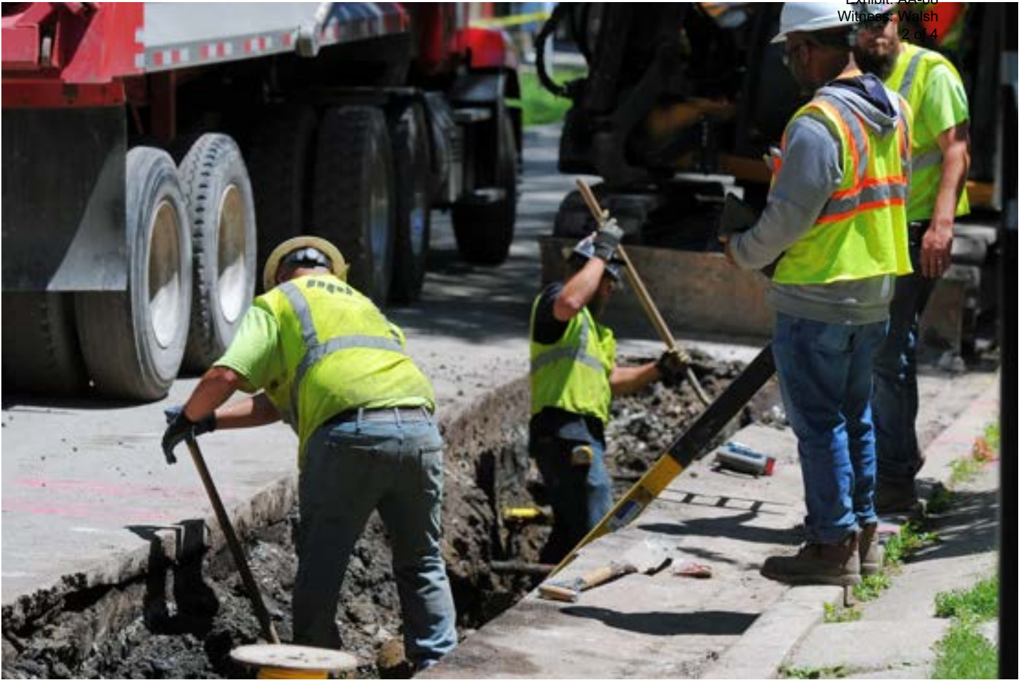
Peoples Gas workers installing a new natural gas pipe in Albany Park in 2019. The utility is replacing deteriorating gas pipes under a program that's scheduled to take until 2040 to complete. | VICTOR HILITSKI / SUN-TIMES FILE
