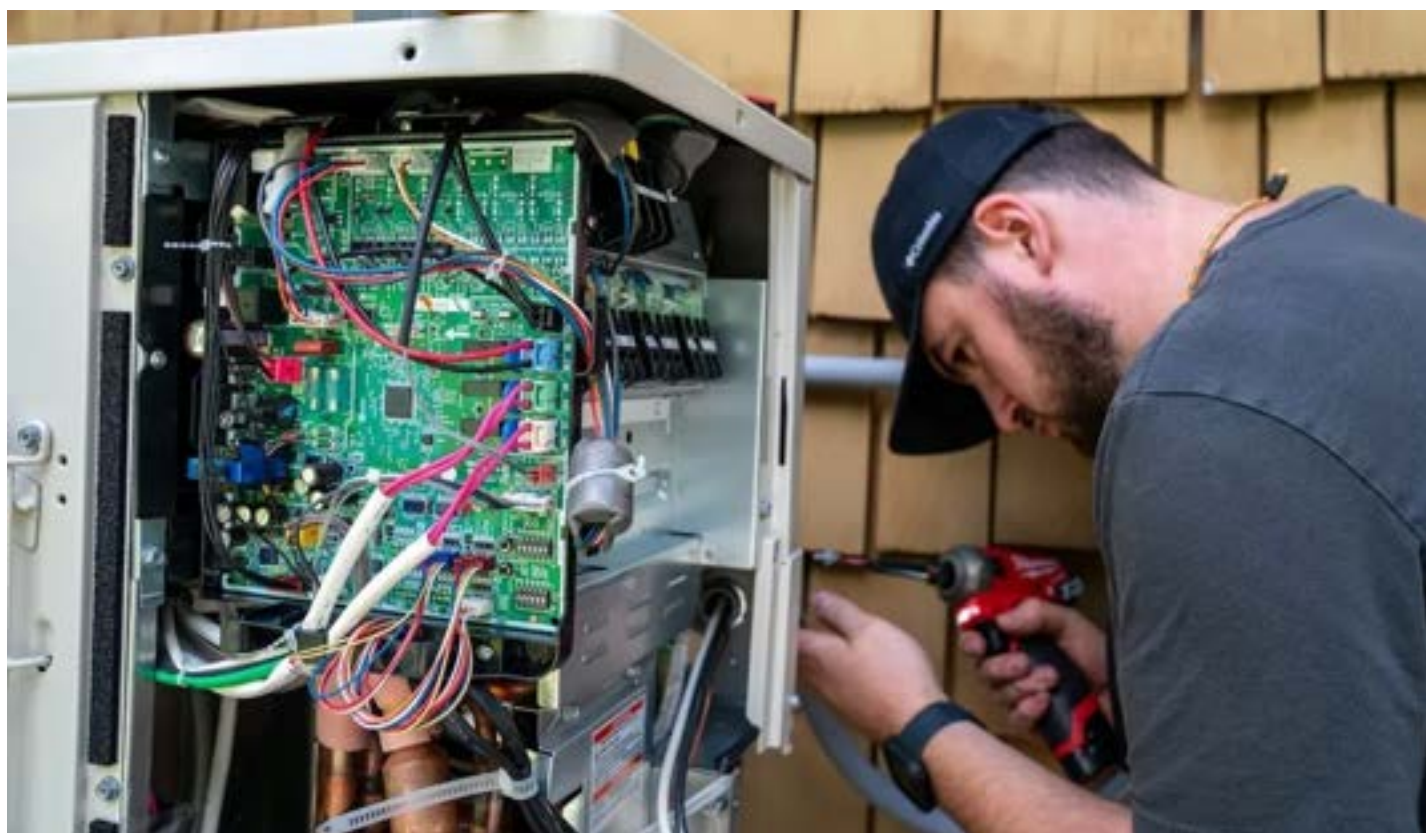
An electrician installs a heat pump on July 21, 2025, in Charlotte, Vermont. (Robert Nickelsberg/Getty Images)
