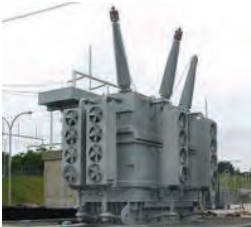
Figure 2. Typical Step-Up transformer
