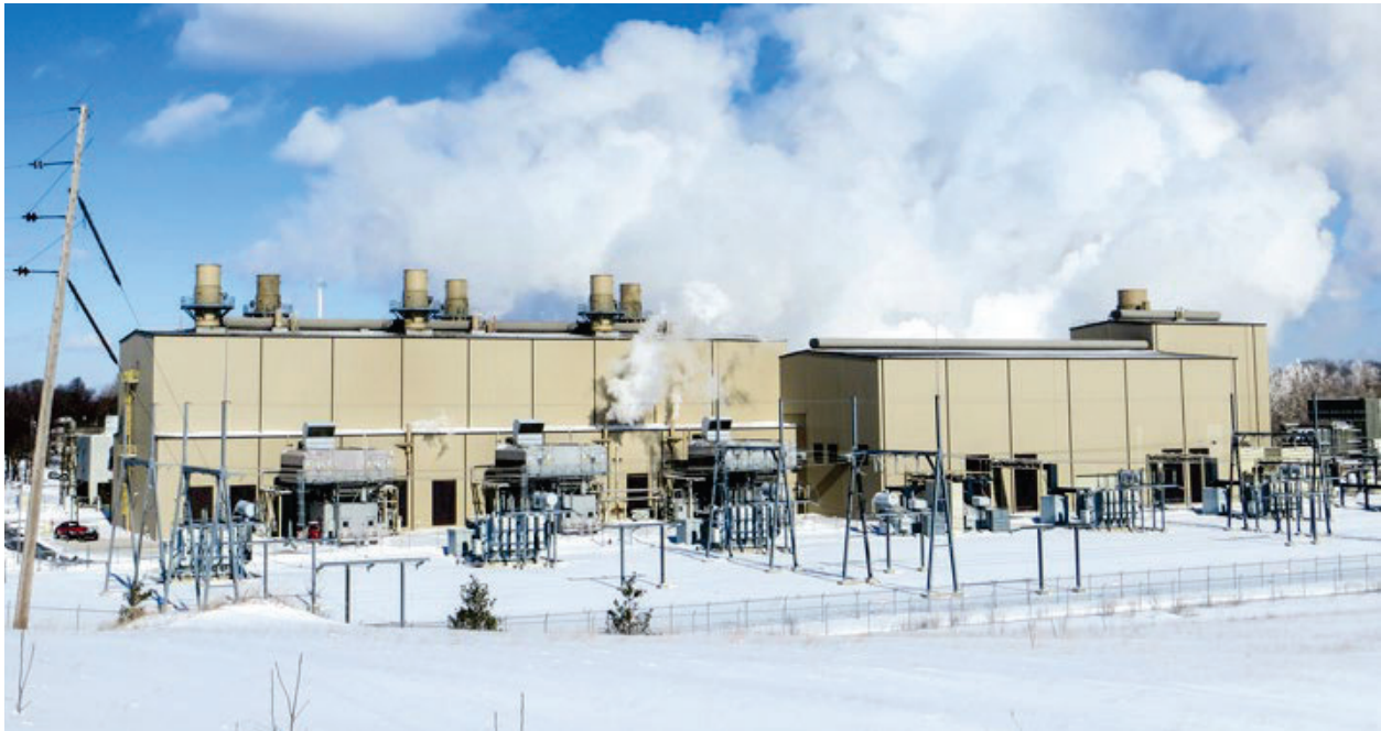
Figure 1. Jackson Generating Station.
