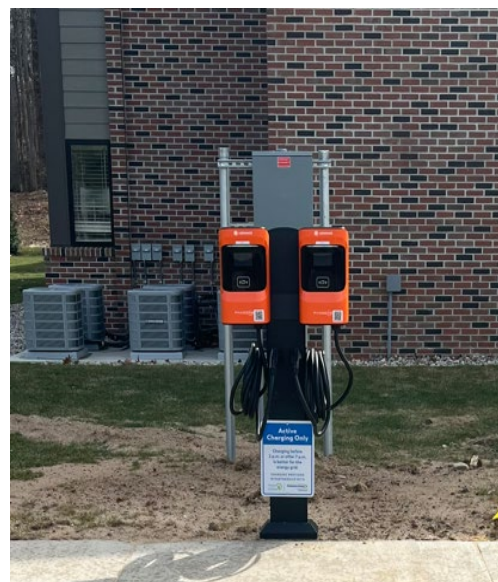
PowerMIDrive Multifamily Property Charging in Wyoming, MI
