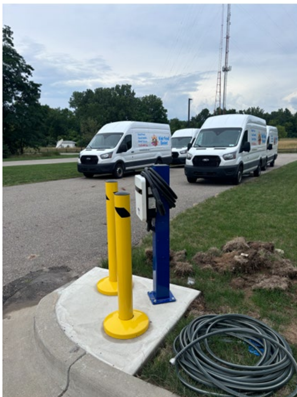
L2 charging infrastructure being installed for Kids Food Basket and made possible via the enhanced rebates for income-qualified fleets
