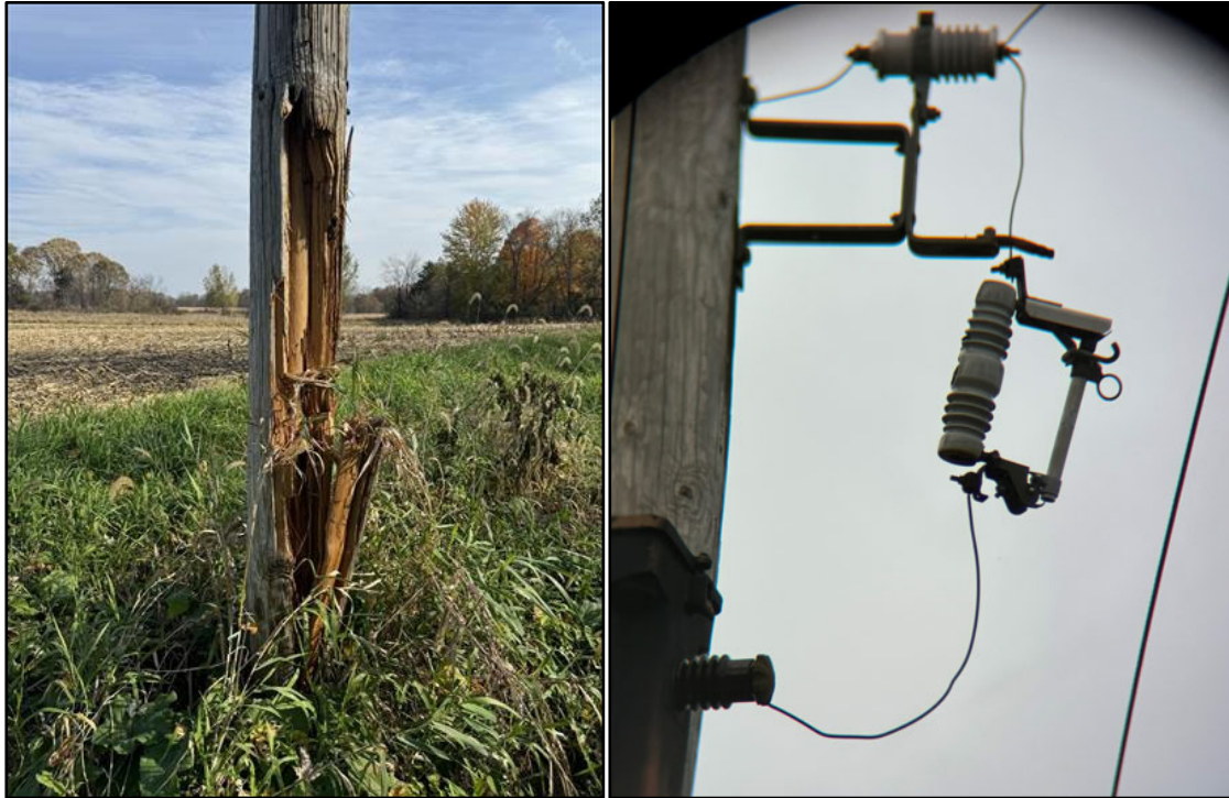
FIGURE 10 LVD P2 FAILURES IDENTIFIED THROUGH SECURITY ASSESSMENTS
