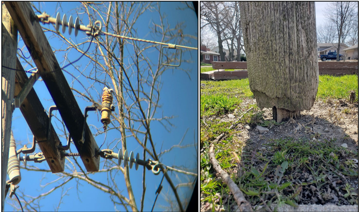
FIGURE 9 LVD P2 FAILURES IDENTIFIED THROUGH SECURITY ASSESSMENTS
