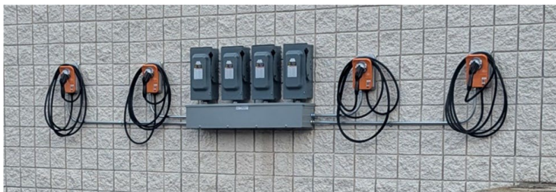
Fleet charging setup at a rental car agency
