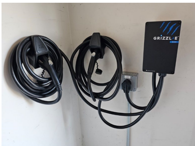
A home charging setup for two EVs from a single NEMA 14-50 outlet offers power sharing for optimal load management as more homes adopt a second and third EV
