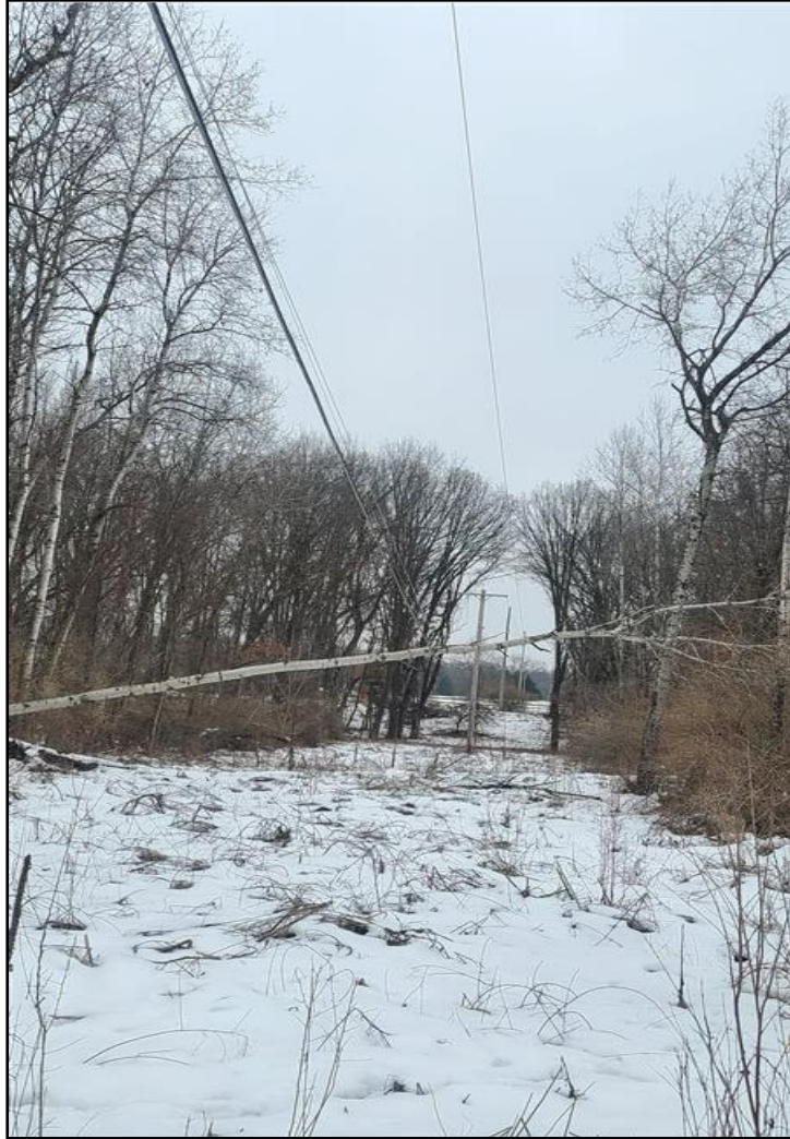
FIGURE 50 TREE ON OVERHEAD SINGLE-PHASE PRIMARY LINE
