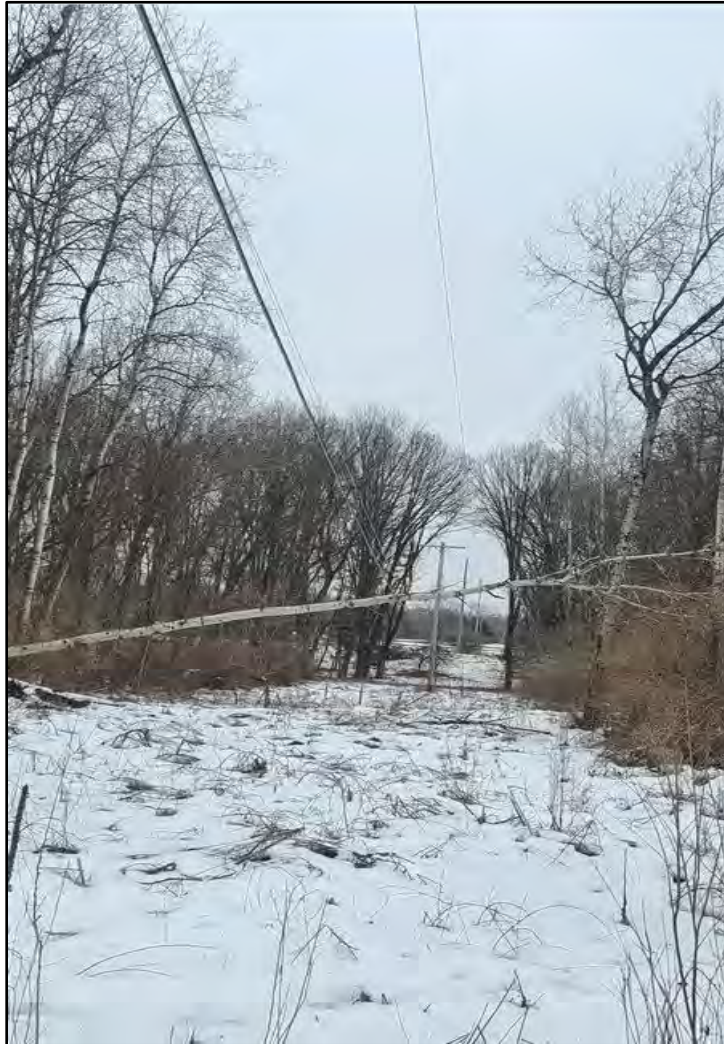
FIGURE 50 TREE ON OVERHEAD SINGLE-PHASE PRIMARY LINE
