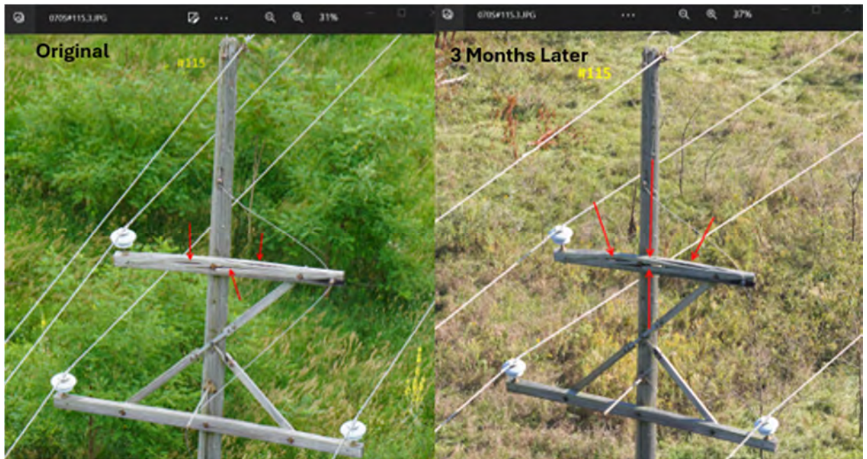
FIGURE 19 PRIORITY 3 CROSS ARM 3-MONTH DETERIORATION
