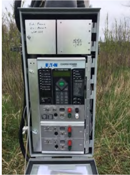
FIGURE 6 VOLTAGE REGULATOR CONTROLLER
