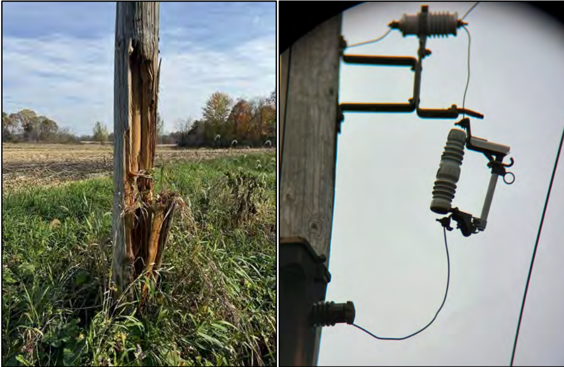
FIGURE 10 LVD P2 FAILURES IDENTIFIED THROUGH SECURITY ASSESSMENTS
