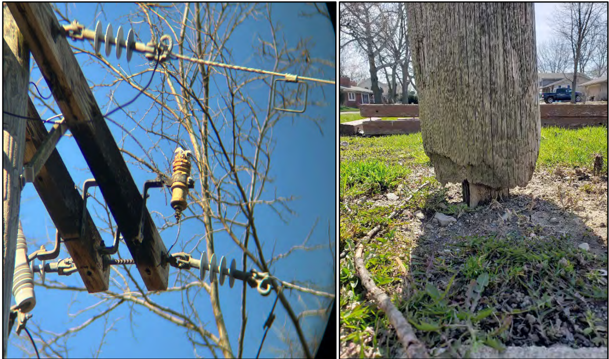
FIGURE 9 LVD P2 FAILURES IDENTIFIED THROUGH SECURITY ASSESSMENTS
