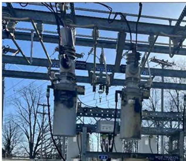
FIGURE 36 DAMAGE FROM ANIMAL CONTACT
