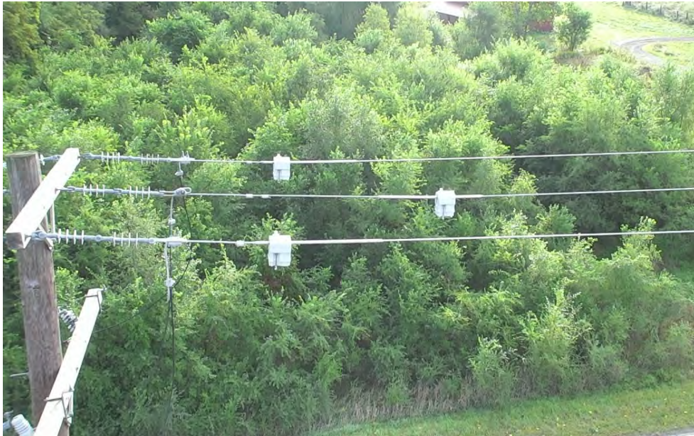
FIGURE 4 3-PHASE LINE SENSOR INSTALLATION
