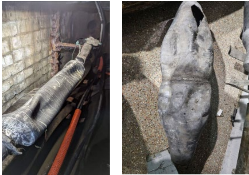
Figure 11 Swollen and Leaking Lead Sleeves
