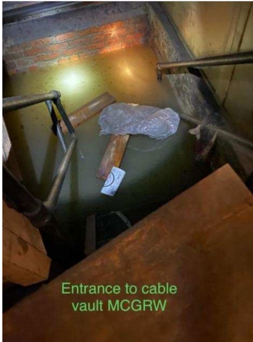
Figure 13. McGraw Substation Flooding – Stairway to Sub-Grade Portion of Station
