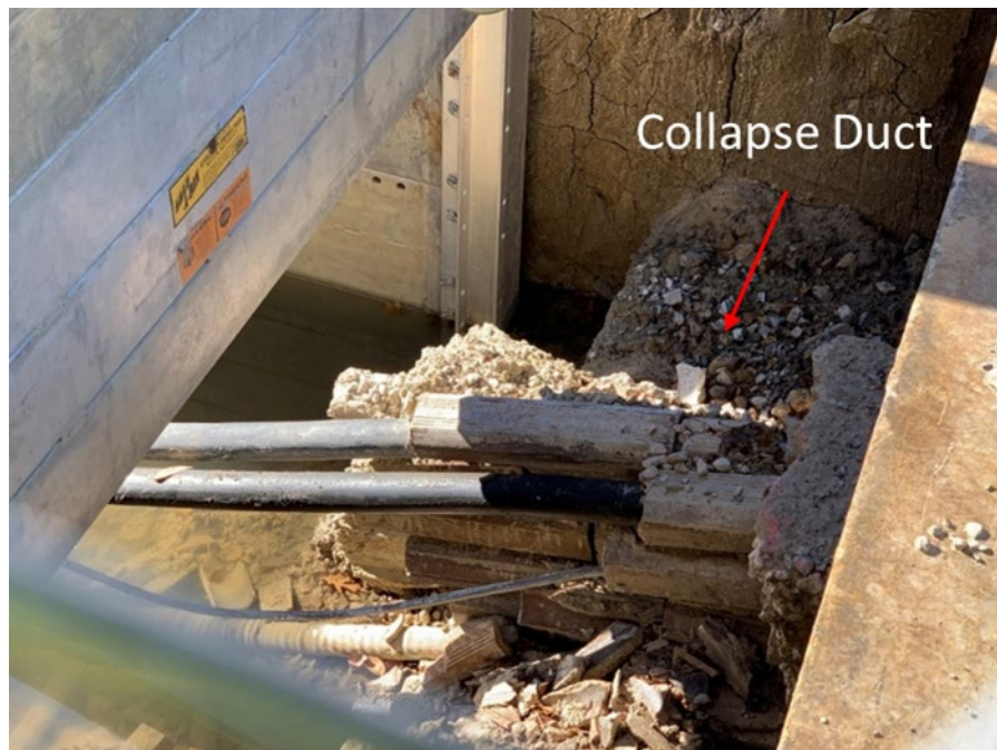
9 Figure 9. System Cable – UG Collapsed Duct
