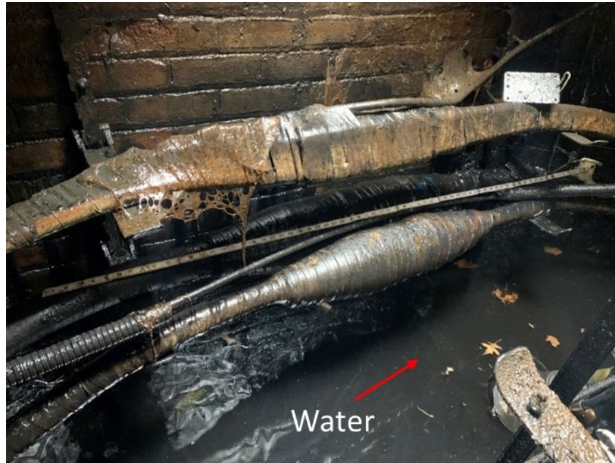
Figure 10. System Cable – Cable Inside Manhole
