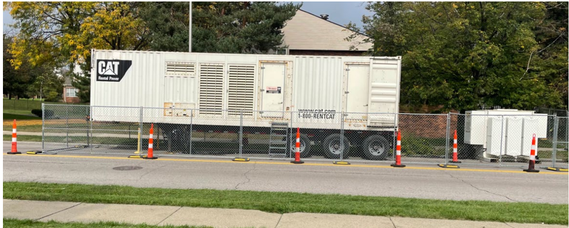
Figure 23 Representative Example Portable Generator Utilized on TRK0359
