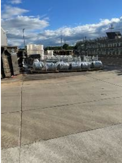
Jackson wire, transformers, switches
