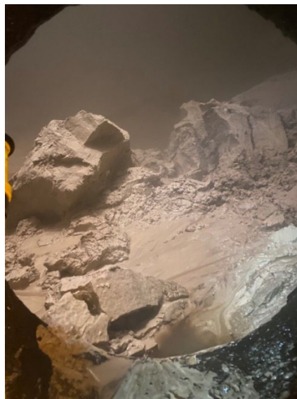
Figure 2 – Solidified Slurry in the Filter Feed Tank following over four shifts of High-Pressure Cleaning and Vacuuming
