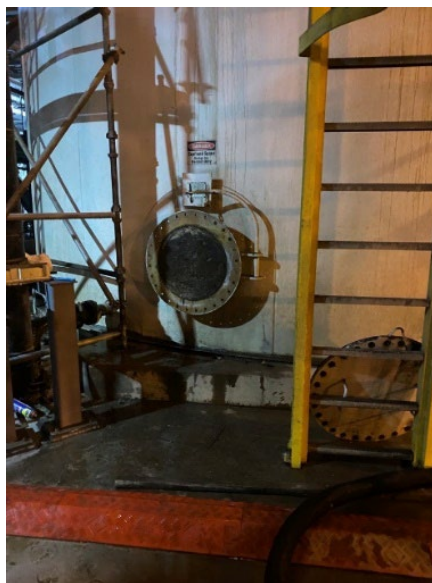
Figure 1 – Filter Feed Tank Manhole Access Door with severe pluggage
