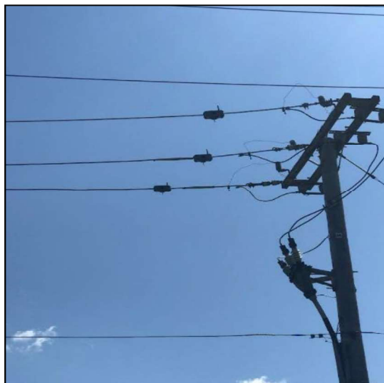
Location of the Smart Fault Indicators
