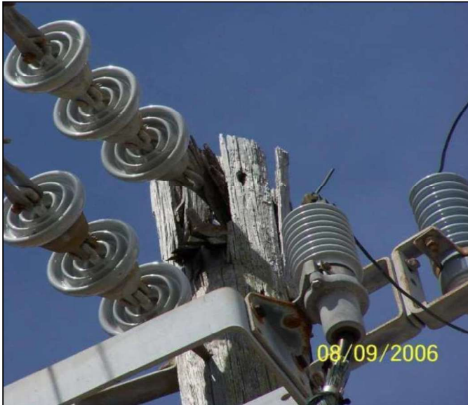
Defective Pole Top
