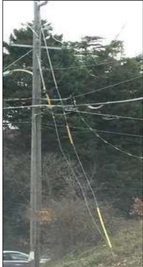
Defective Guy Wire
