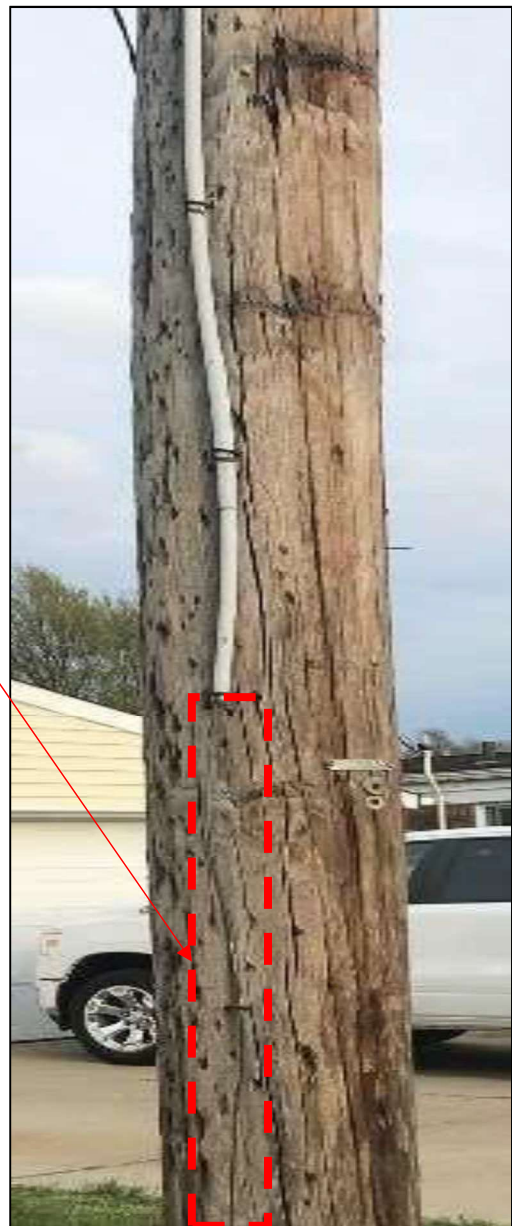
Defective Ground Wire (non-continuous)
