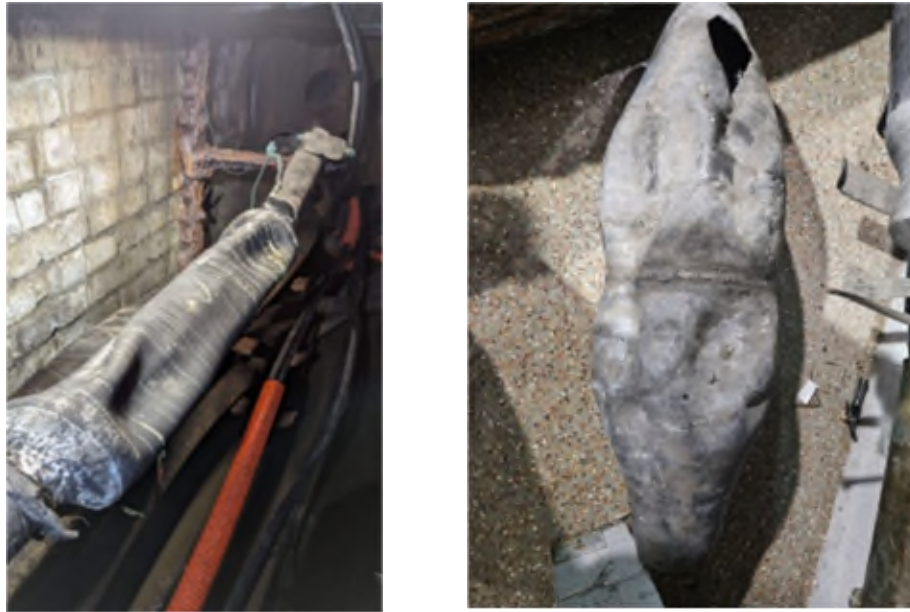
Figure 5 Leaking & swollen sleeve examples
