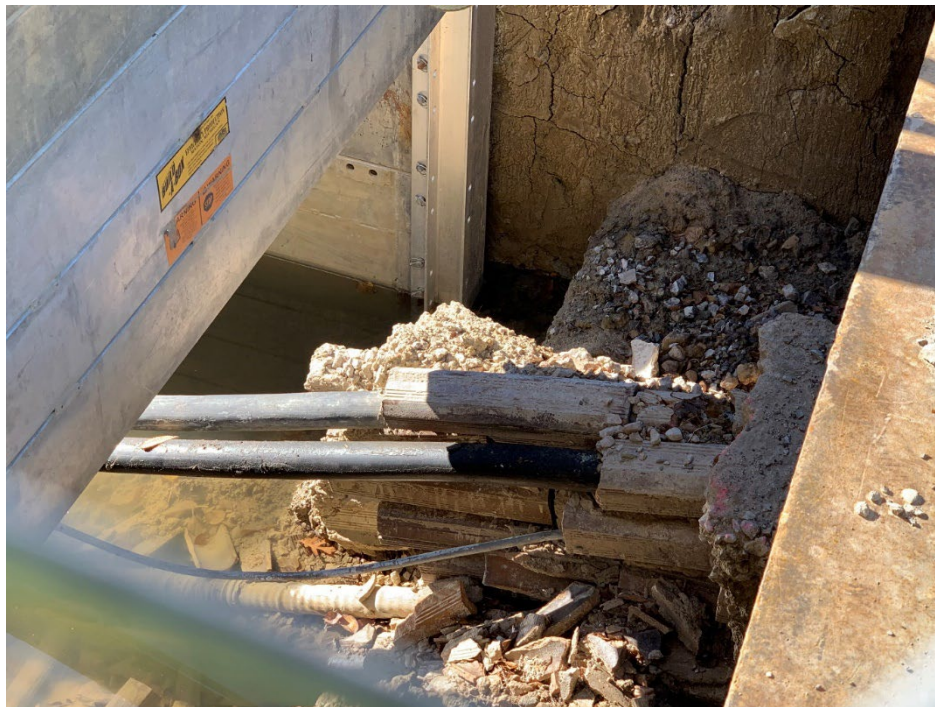
8 9 Figure 23. System Cable – UG Collapsed Duct
