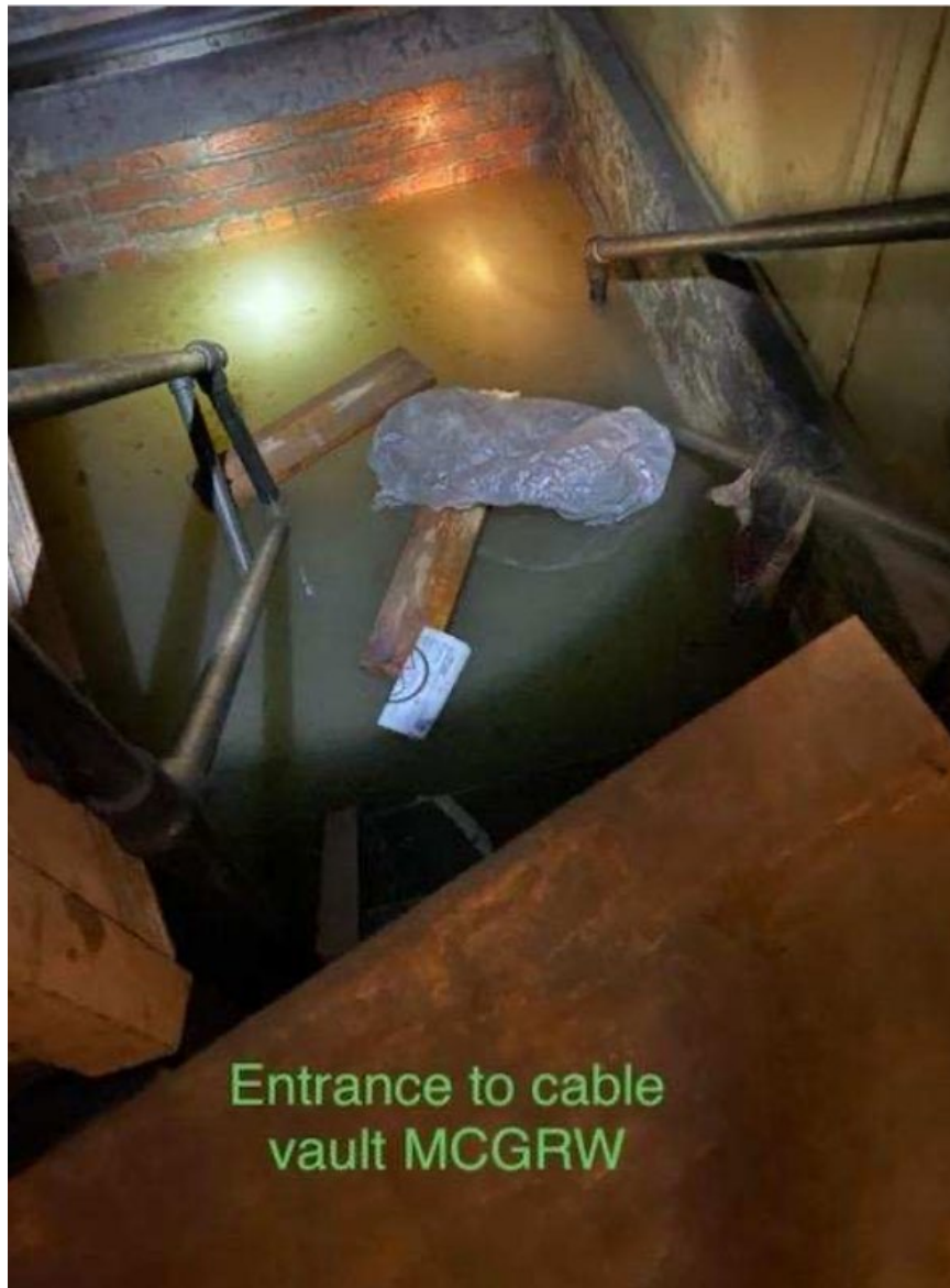
Figure 17. McGraw Substation Flooding – Example 1
