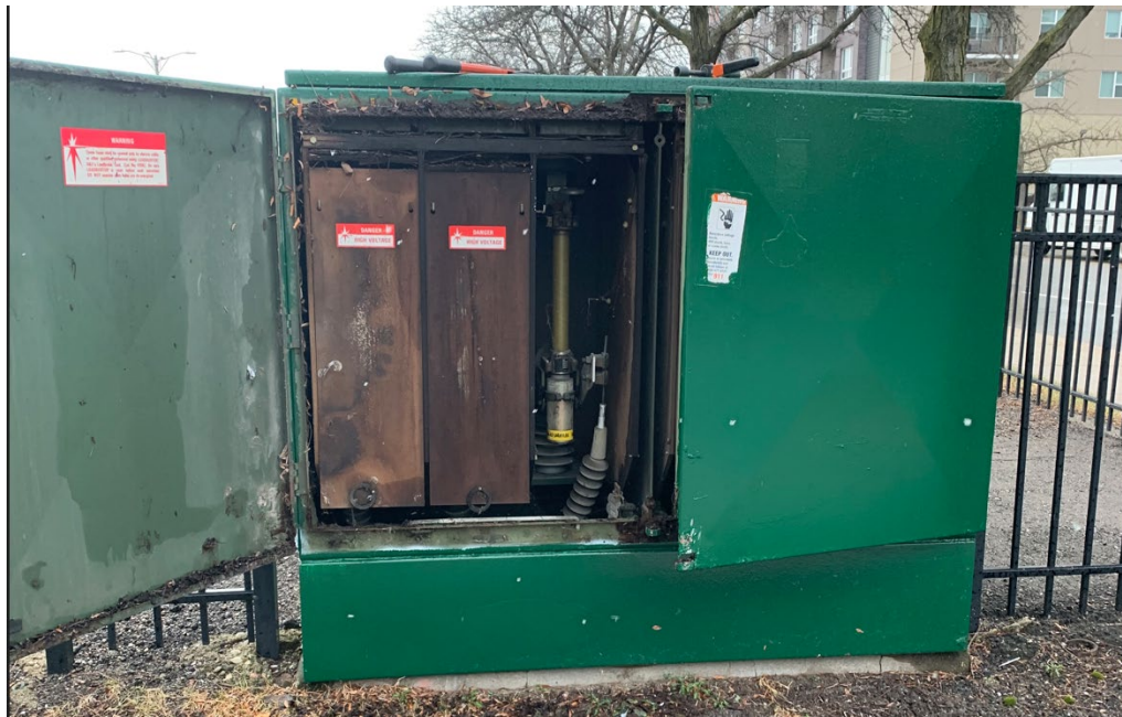
Figure 27. Live-front UG Transformer
