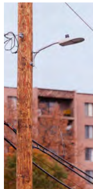
DTE Wood Poles: Existing distribution poles or new 30' wood poles
