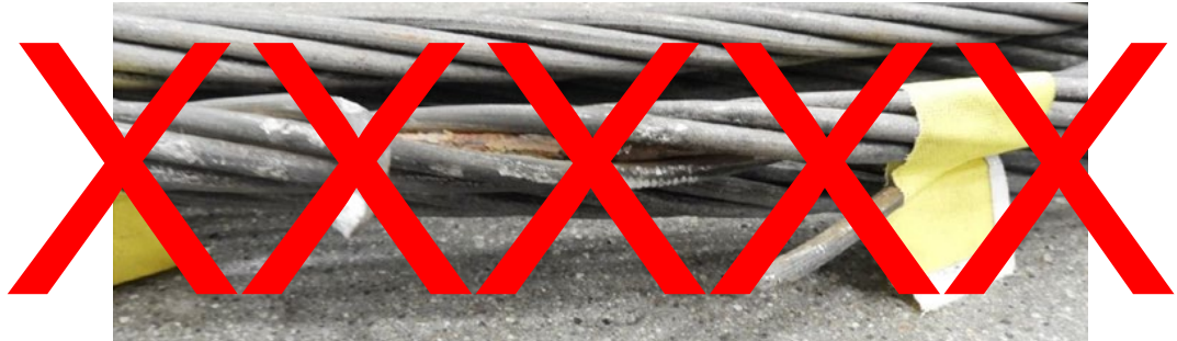
Figure 9: Existing Tie 4105 3/0 ACSR reduced tensile strength
