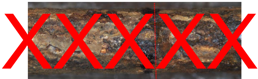
13 Figure 8 : Existing Tie 4105 Steel Core of 3/0 ACSR conductor showing 14 corrosion
