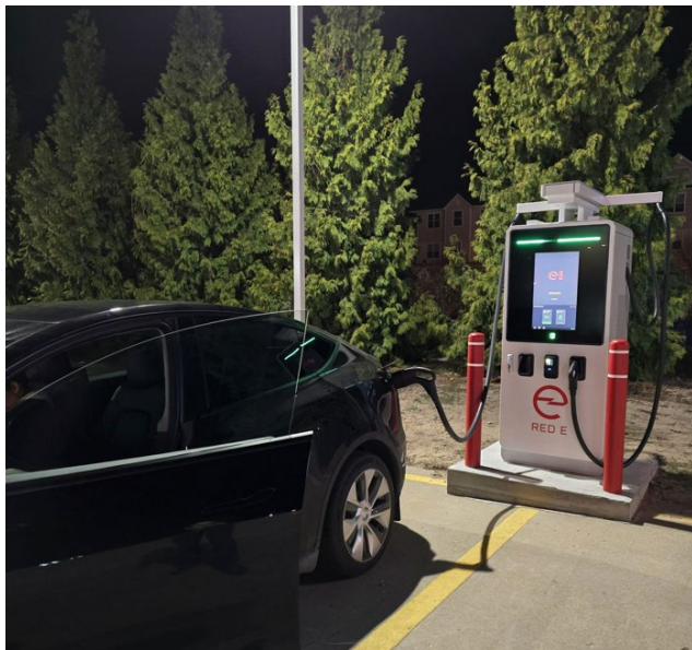
A DCFC in Ludington provides nighttime charging for travel along Michigan's west coast
