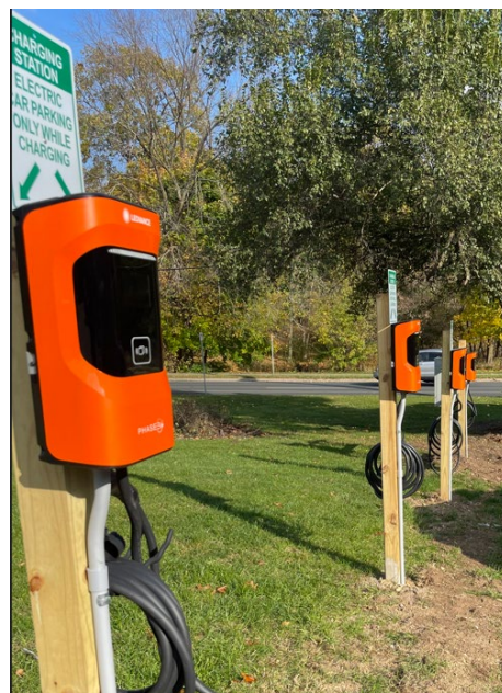
PowerMIDrive Multifamily Property Charging in Kalamazoo
