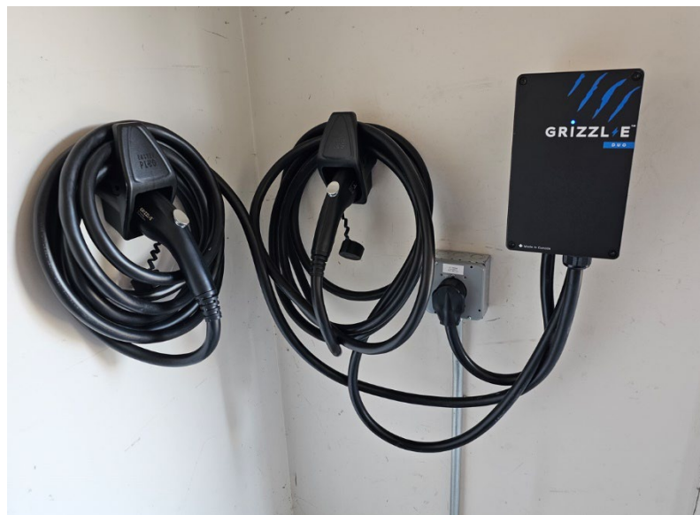
A home charging setup for two EVs from a single NEMA 14-50 outlet offers power sharing for optimal load management
