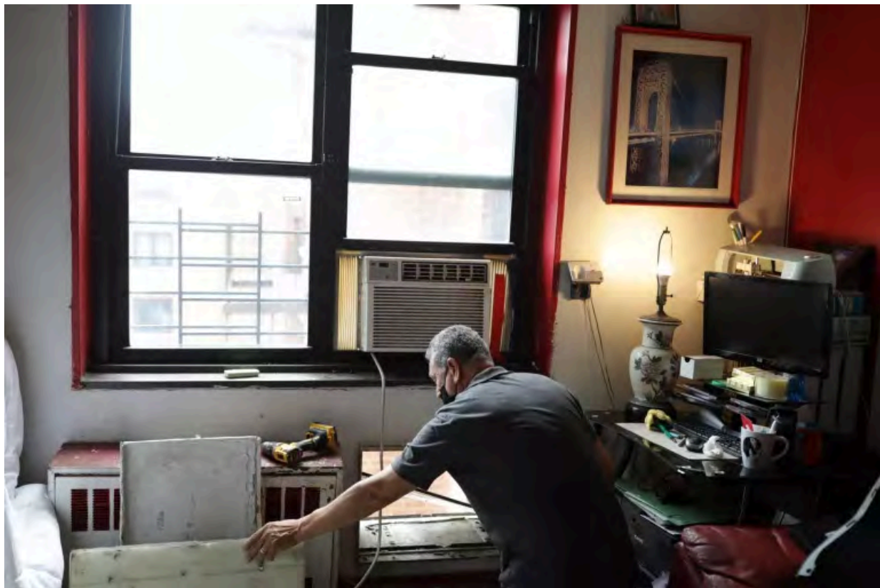
An Association for Energy Affordability crew member works on a weatherization project at an apartment in New York City. | Natalie Keyssar for NRDC
