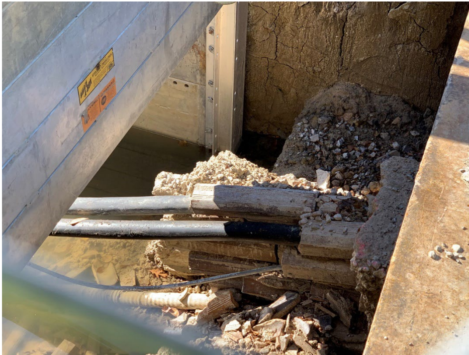
Figure 23. System Cable – UG Collapsed Duct
