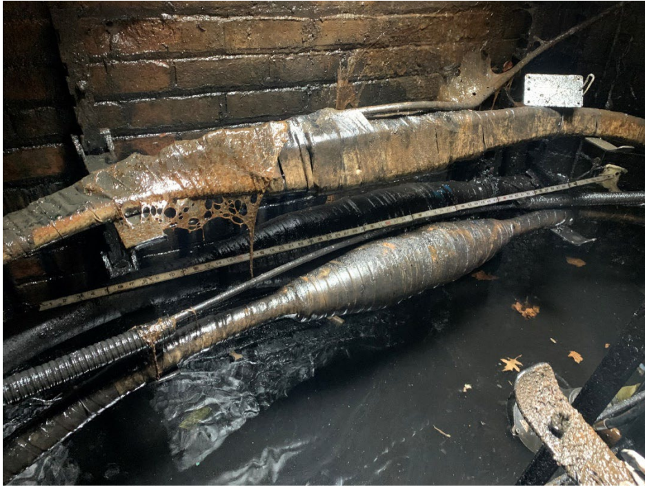
Figure 24. System Cable – Cable Inside Manhole
