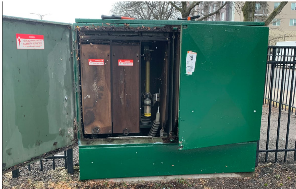
Figure 27. Live-front UG Transformer
