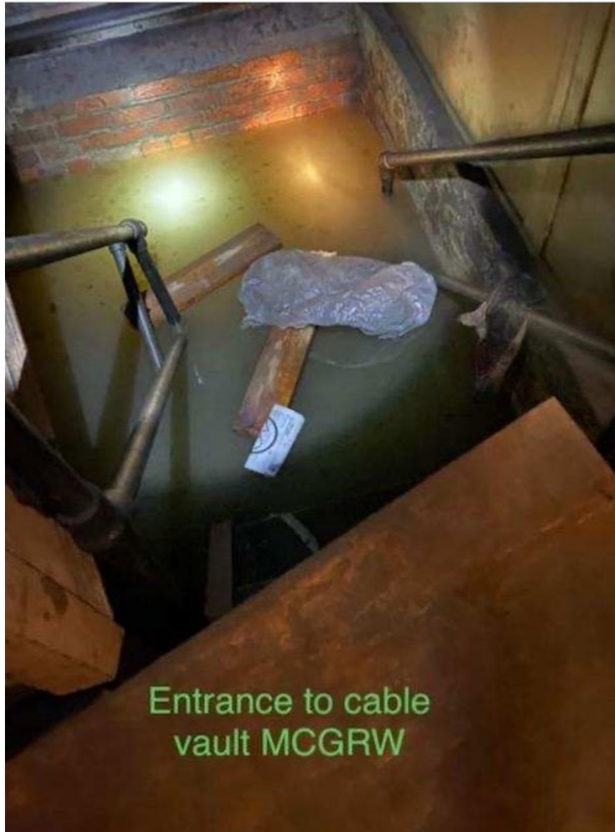
Figure 17. McGraw Substation Flooding – Example 1
