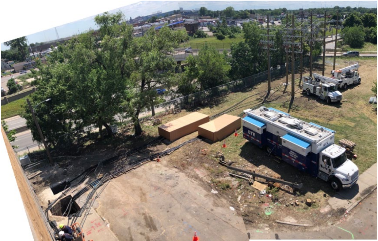
Figure 19. McGraw Substation – Temporary Pole Farm
