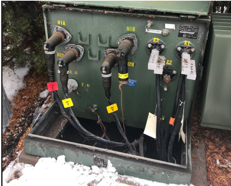
Figure 28. Dead-front UG Transformer
