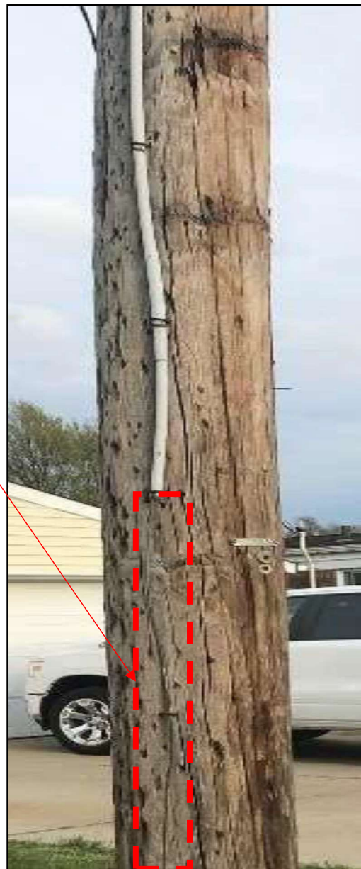
Defective Ground Wire (non-continuous)
