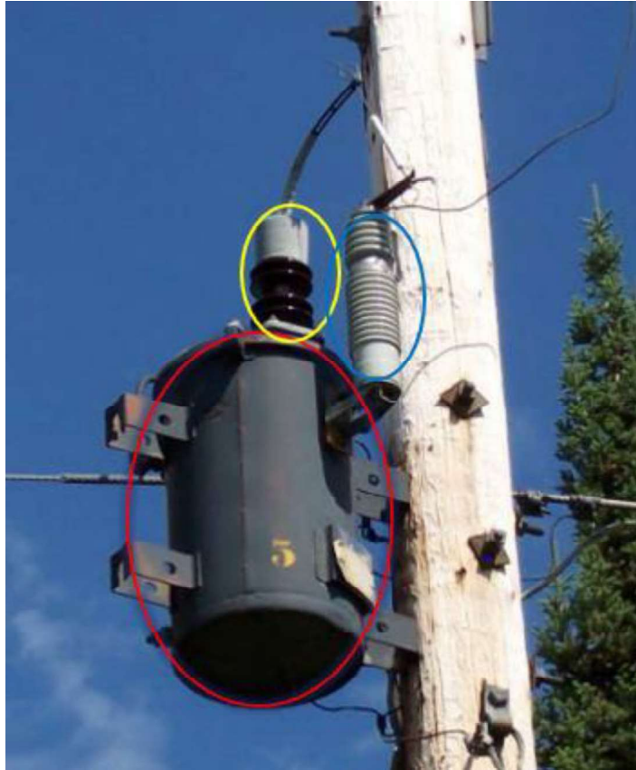
An example of a dark shaded transformer with porcelain insulators that have a shine during daylight.
