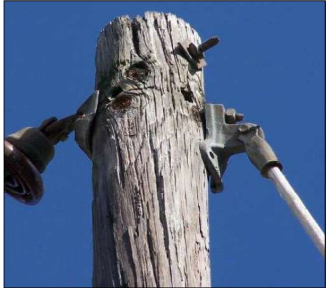
Acceptable Pole Top
