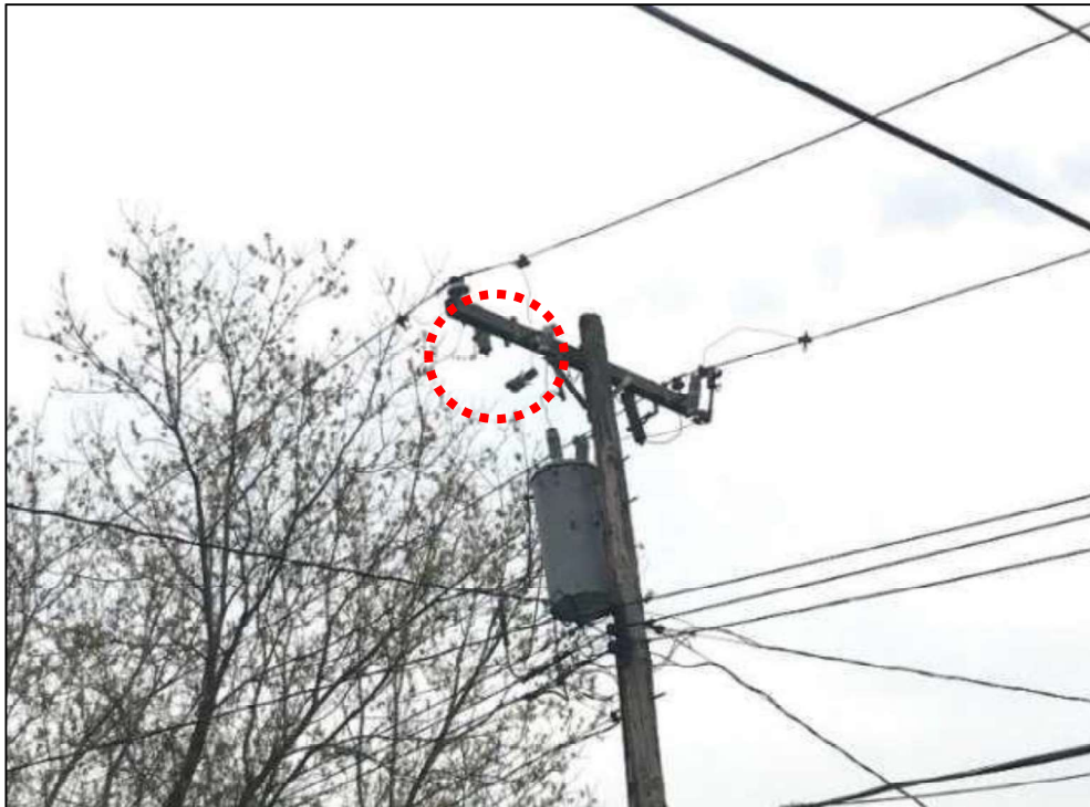
Broken S&C Porcelain cutout just above the transformer
