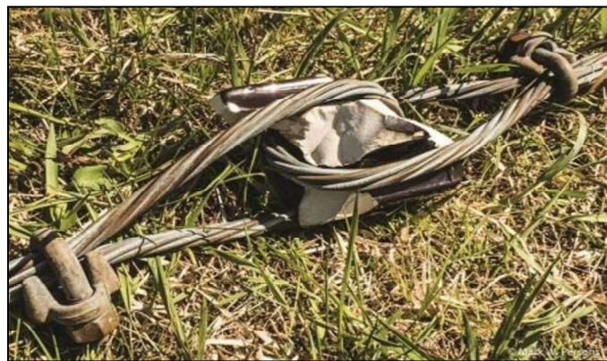
Defective Johnny Ball
