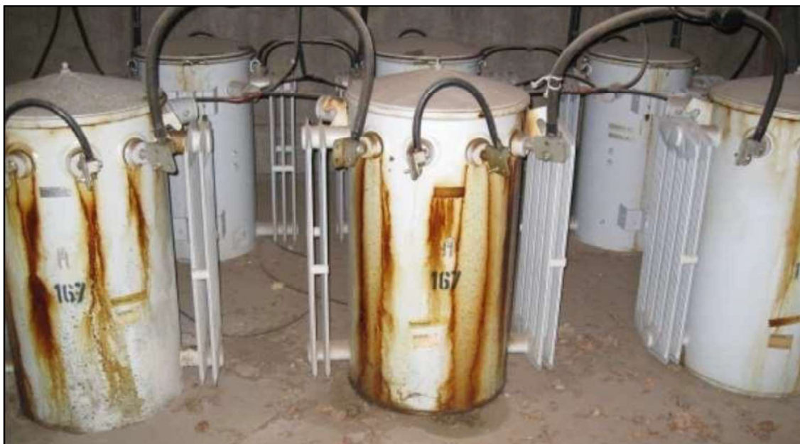
Transformers with Oil Leakage to be reported immediately.
